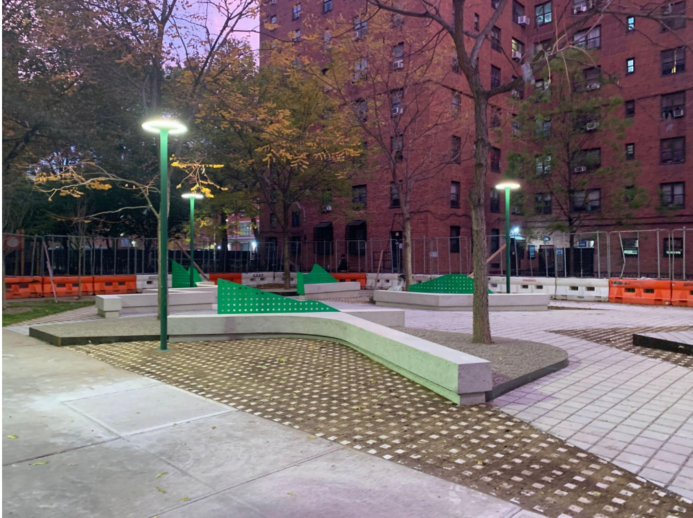
Final stages of construction ahead of the 11/12 ribbon cutting, courtesy of Davies Toews.
